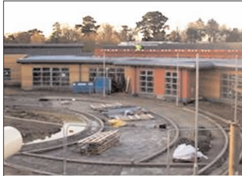
Taking shape: The hospital for which Fareham has waited over three decades.
